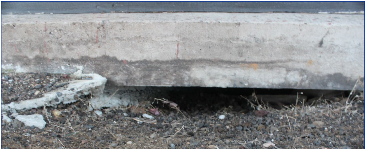
Photo 13: View of a void underneath the concrete slab foundation.
