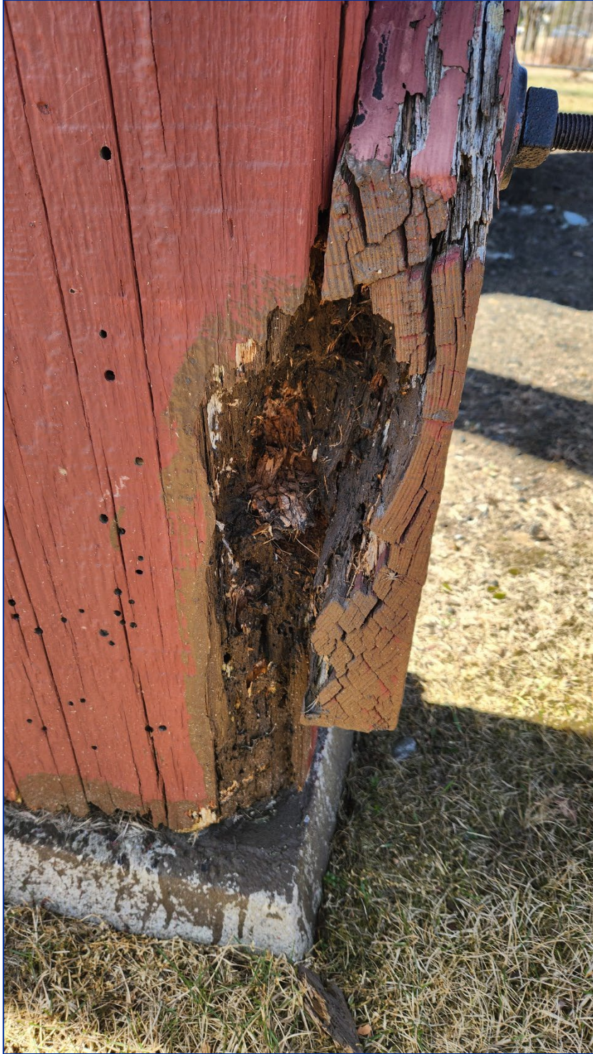
Photo 11: View of damaged and decaying wood timber supports.
