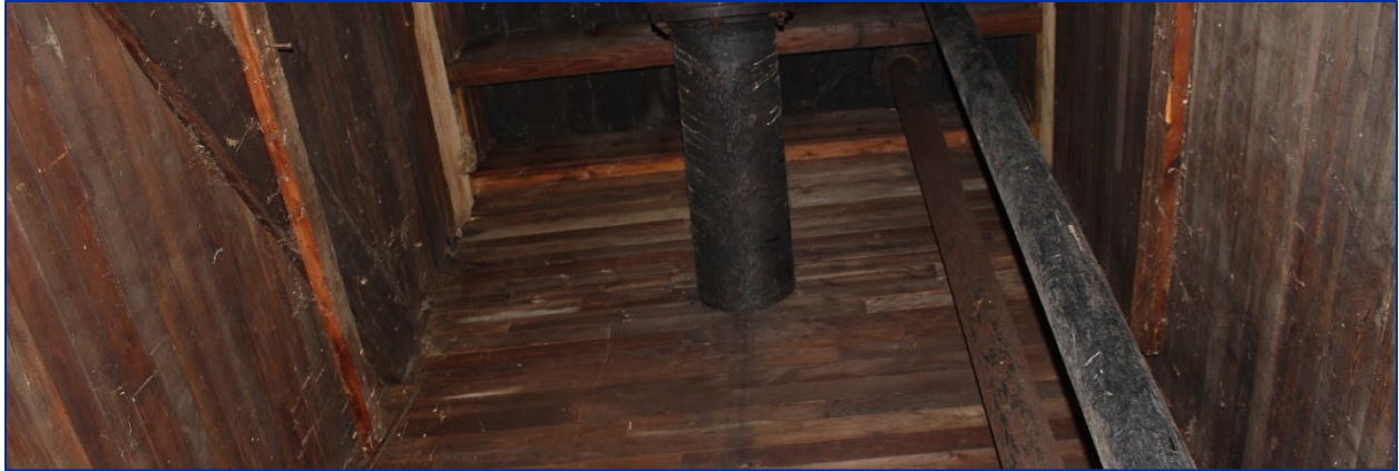
Photo 14: View looking up towards the ceiling with the wood siding and pipe remnants visible.
