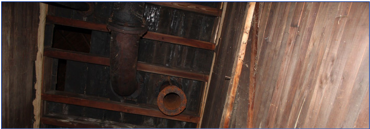
Photo 15: View looking up towards the ceiling with pipe remnants visible.
