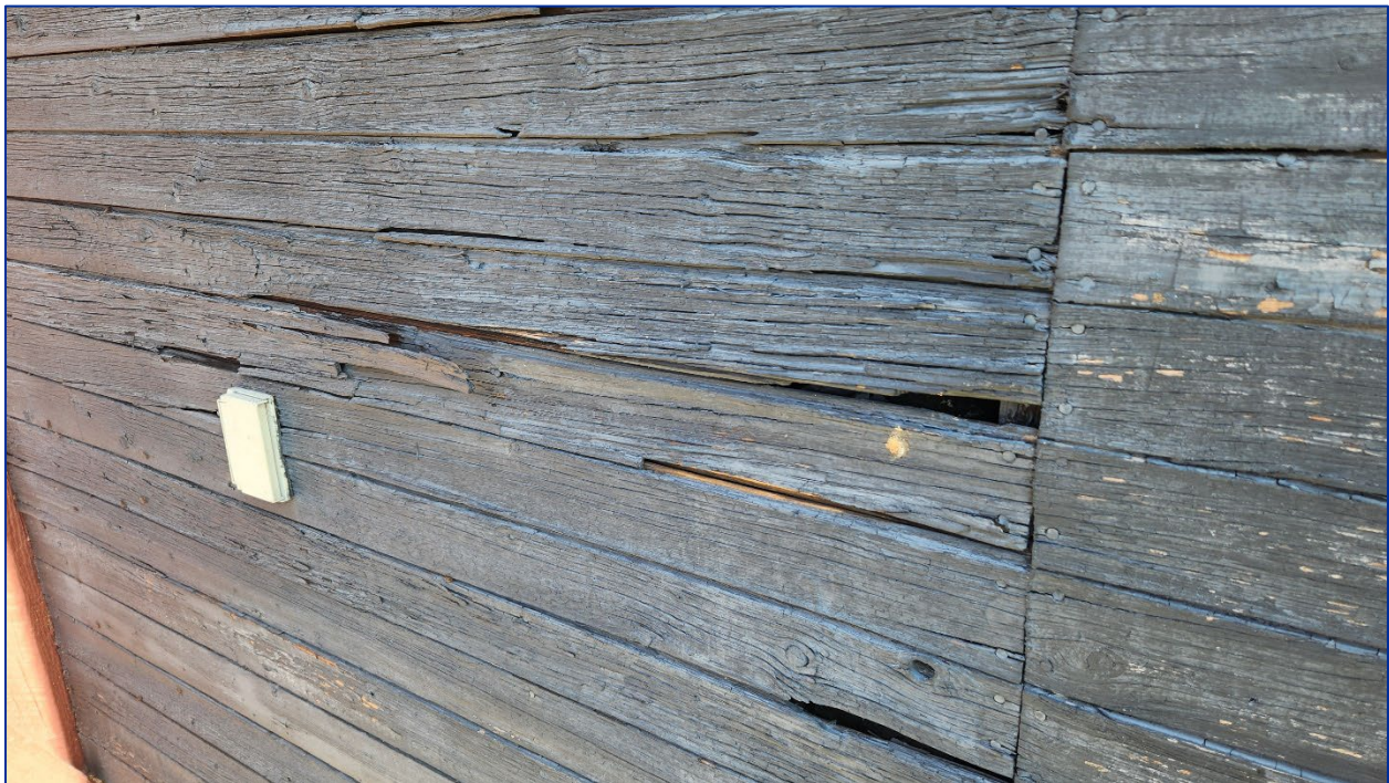
Photo 10: View of the wood siding of the frost box indicating horizontal checking damage.
