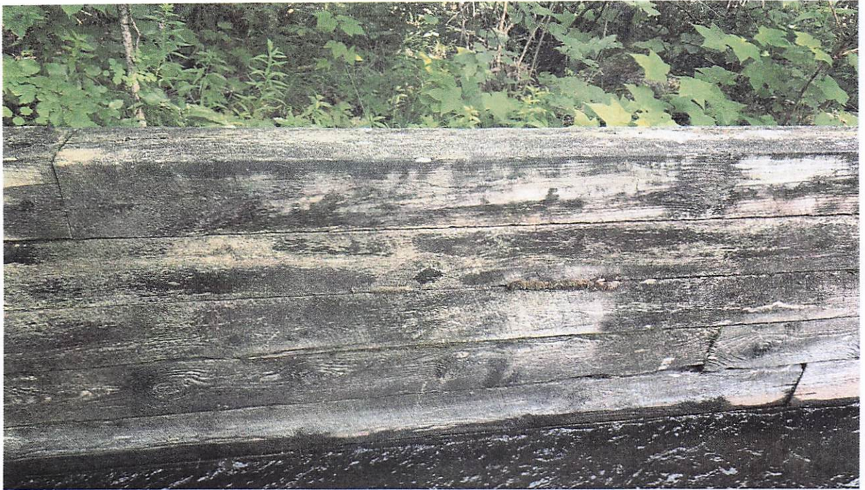
Photo #5: Mid-Section Chute Decay
